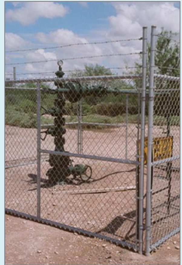
South Weslaco GU#35 wellhead
