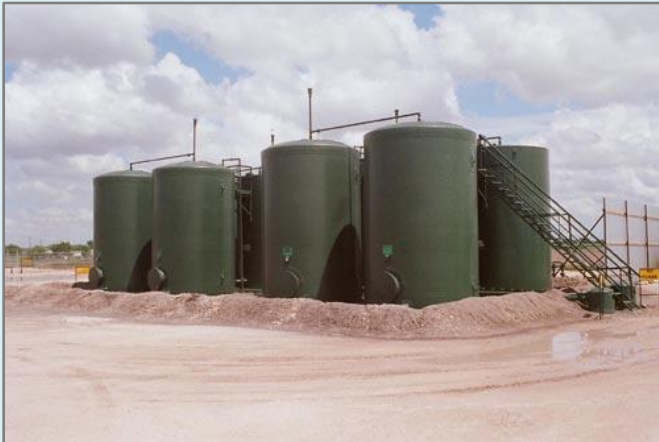
South Weslaco Tank battery
