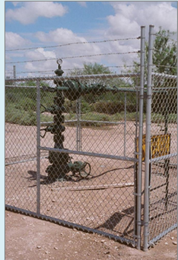
South Weslaco GU-35 wellhead
