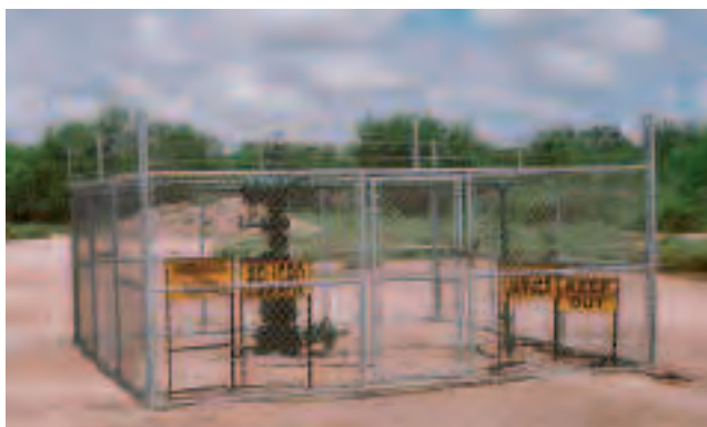
Gas well at South Weslaco
